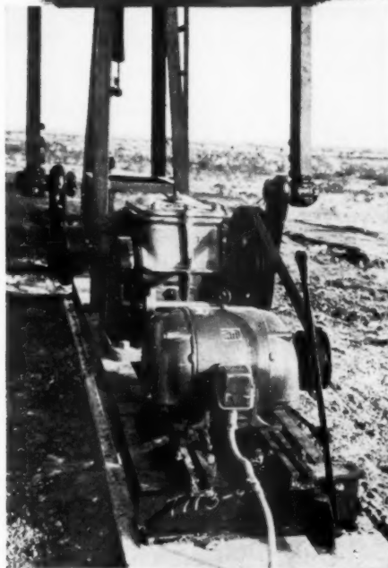
Century 10 horsepower Splash Proof motor driving a pumping unit located in Texas.
